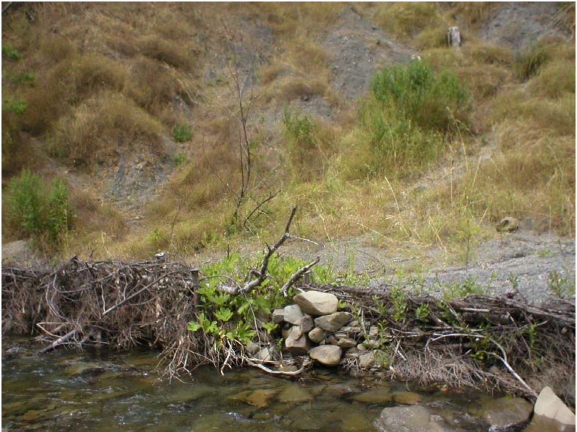
Figure 5. Willow fence at Site 27, nearly one year after installation with willow sprouts, June 28, 2005.
